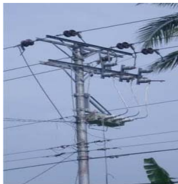
Gambar 6.15 Load Break Switch (LBS)
