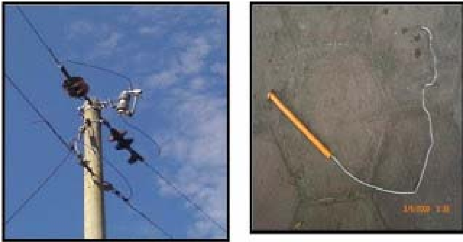
Gambar 6.10 Fuse Cut Out, Fuse Link
