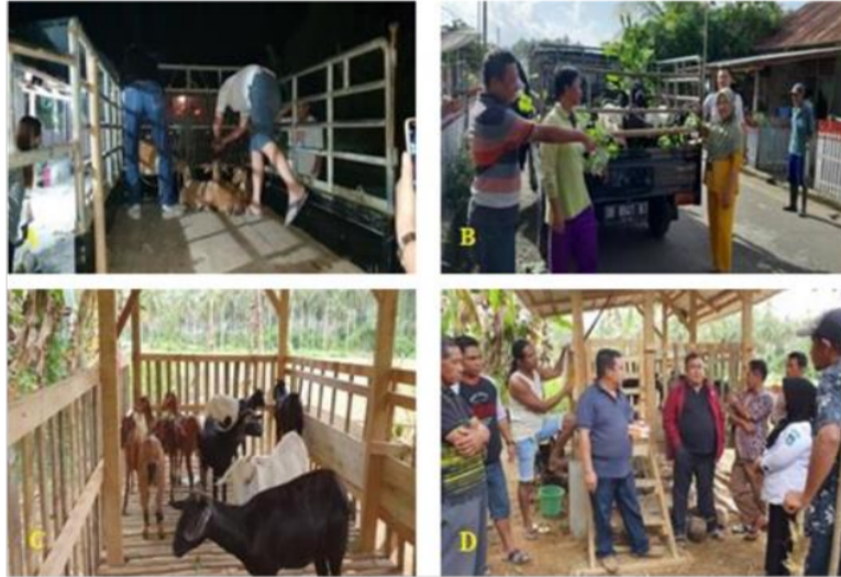
Figure 3. The process of making semi ranch goat pens: A) procurement of materials and tools for making cages; B) installation of cage foundation pole; C) installation of cage roof; and D) completion of cage construction.
